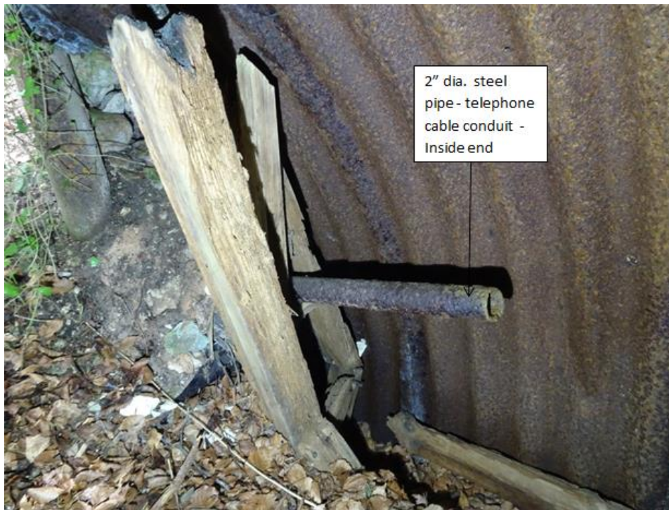
Fig 15 – Telephone cable conduit entry point.
