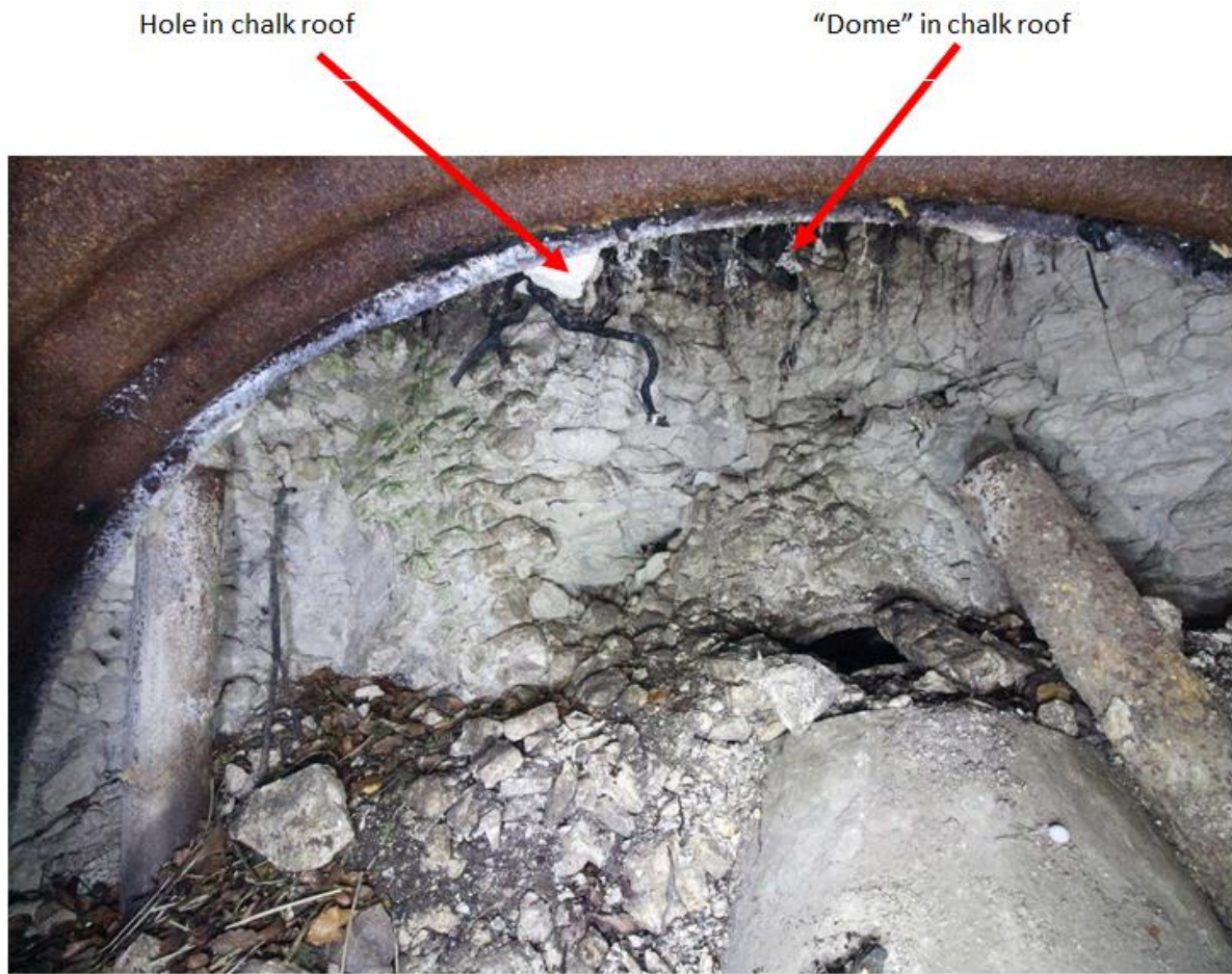
Fig 17 Close up view of back wall showing areas at risk. Also shows two ventilation pipes and two sections of concrete escape tunnel
