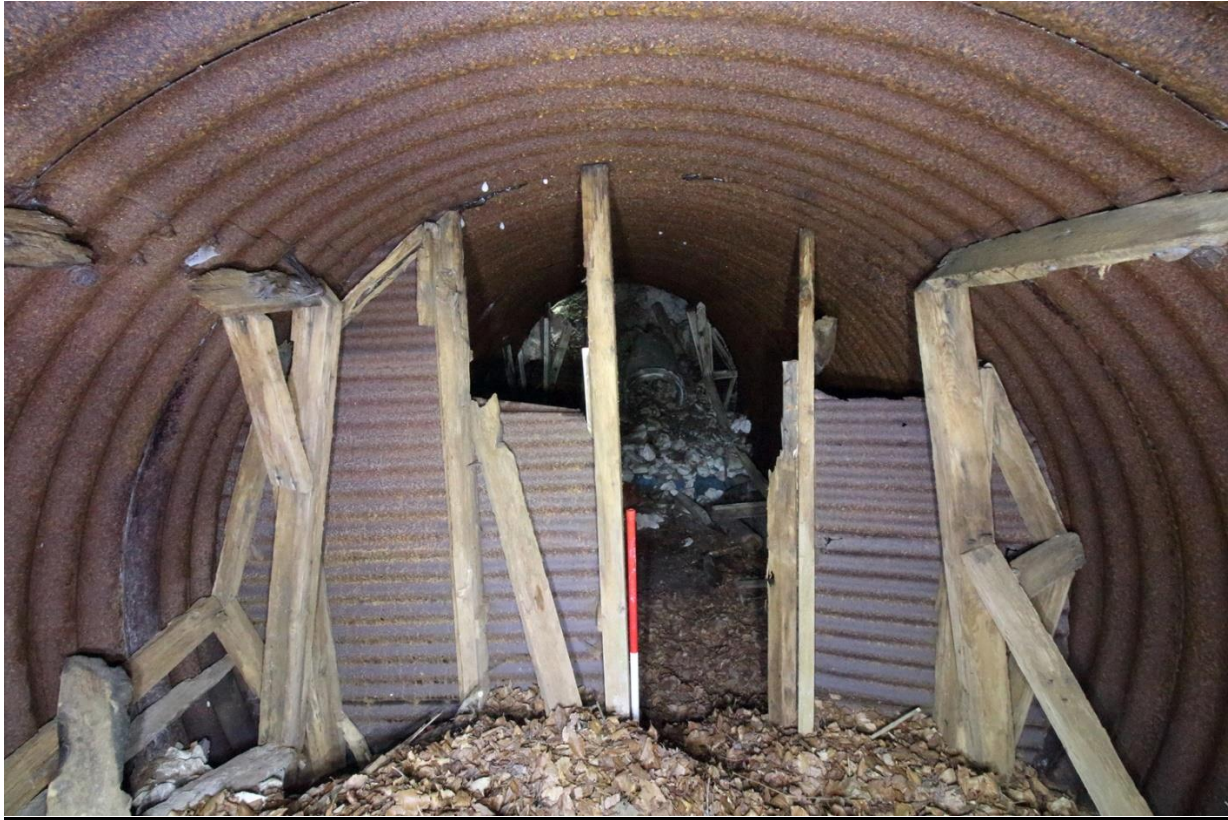
Fig 4 View looking from entrance towards back wall. There would have been a door in the partition but this has been lost
