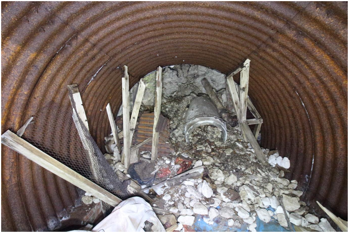
Fig 12 View towards back wall showing construction with 3 sheets of corrugated iron spanning the hideout and the collapsed section of concrete escape tunnel
