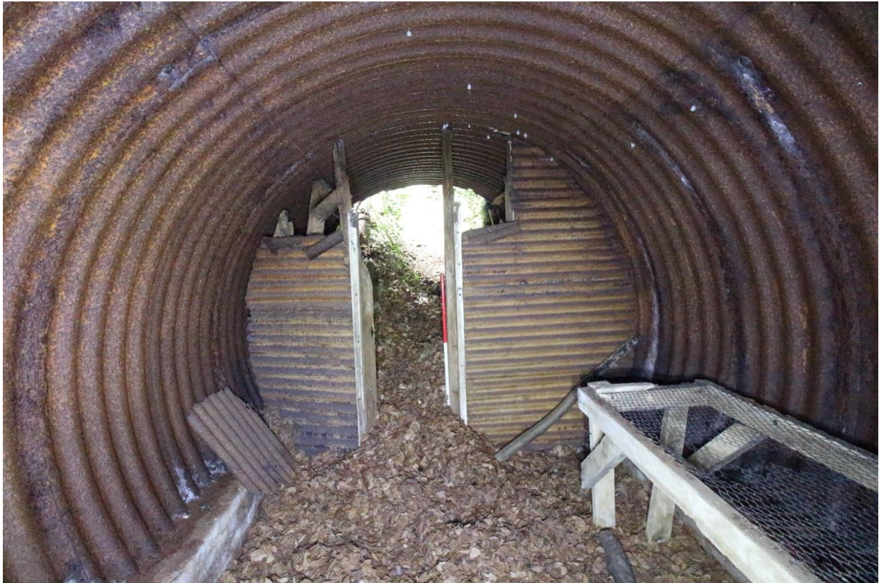
Fig 16 view from back wall towards entrance showing earth spill into entrance
