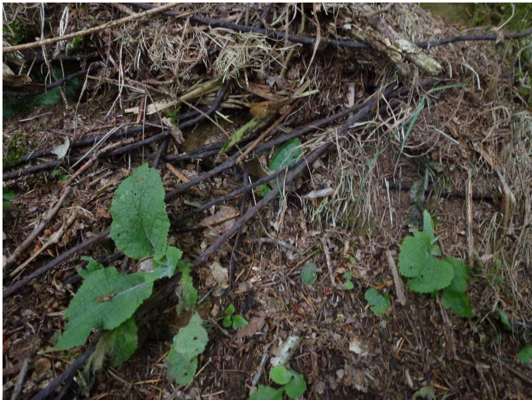
Fig 2. 23 rd September 2013. Multiple strands of rusted metal cable lying parallel exposed on edge of bank.
