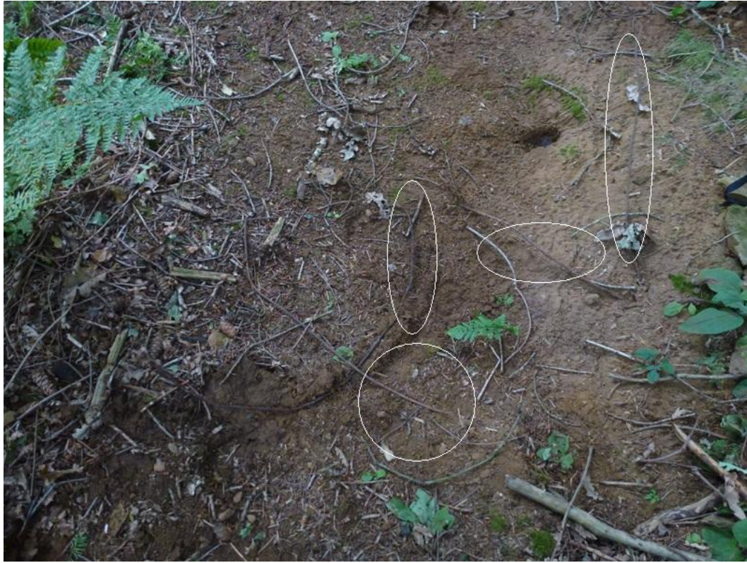
Fig 1. 23 rd September 2013. Lengths of metal cable circled, standing proud of the bank surface following erosion.
