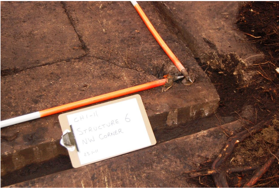
Photo 8: Structure 6 – crack around concrete base, NW corner (Photo No. CH1-11-0022)
