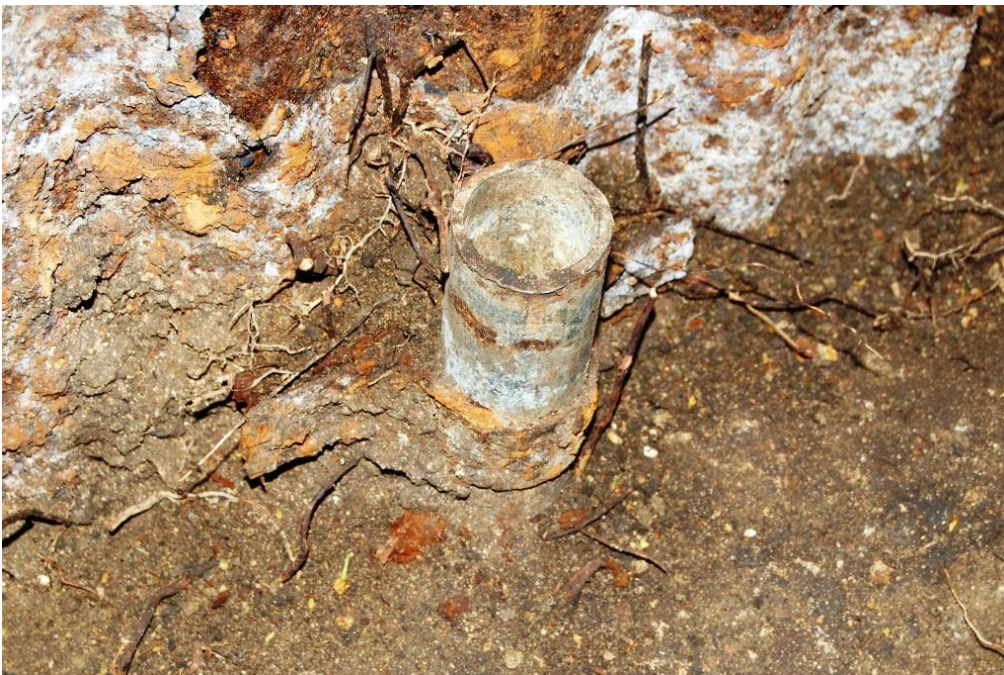
Photo 17: Trench 6 – metal pipe attached to corrugated iron by C bracket (Photo No. CH07-11-0051)
